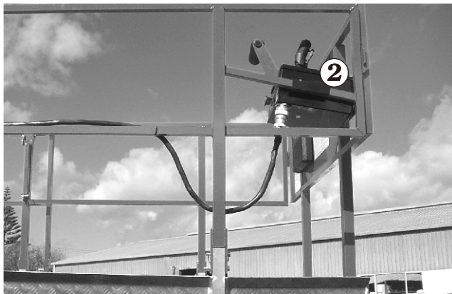
Figure 6.1.2 - Control Box Location, Platform Position
